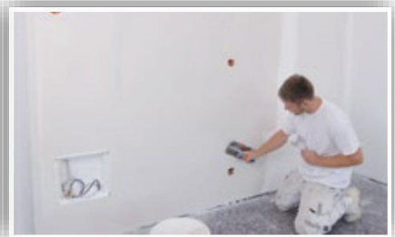
Heating to cover the heating fabric and smoothing the surface with Adheline or Finelime..
